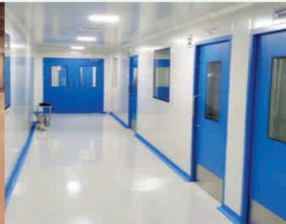
PUF Panel Clean Room
